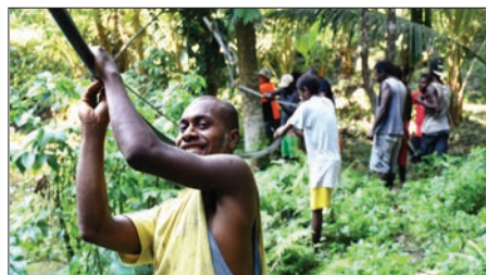
Many village helpers made light of running the new water supply line
